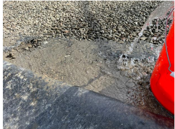
Photo 14 – Water Immediately draining
