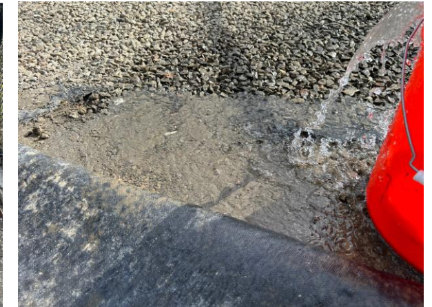
Photo 14 – Water Immediately draining
