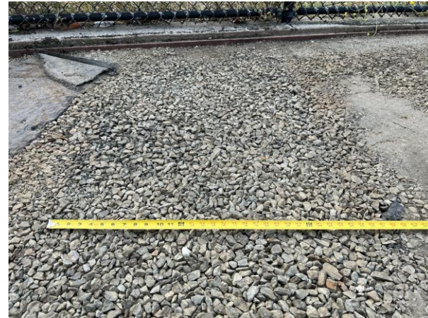
Photo #15 – Infiltration Trench
