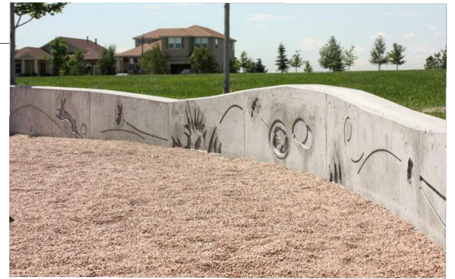
SECURITY WALL AT PLAYGROUND
