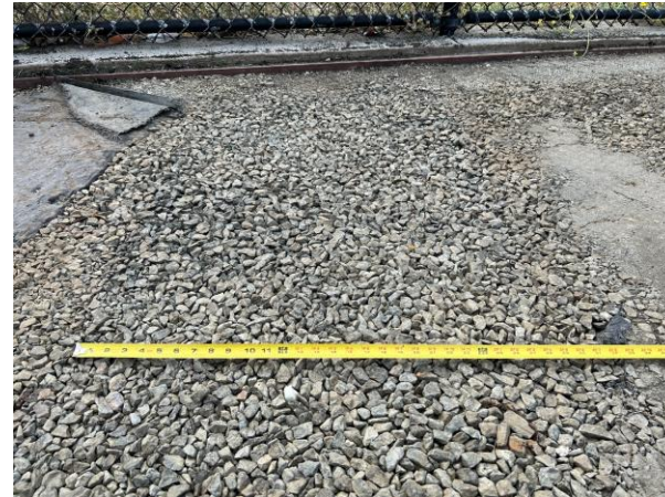
Photo #15 – Infiltration Trench
