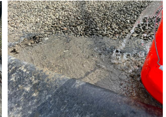
Photo 14 – Water Immediately draining
